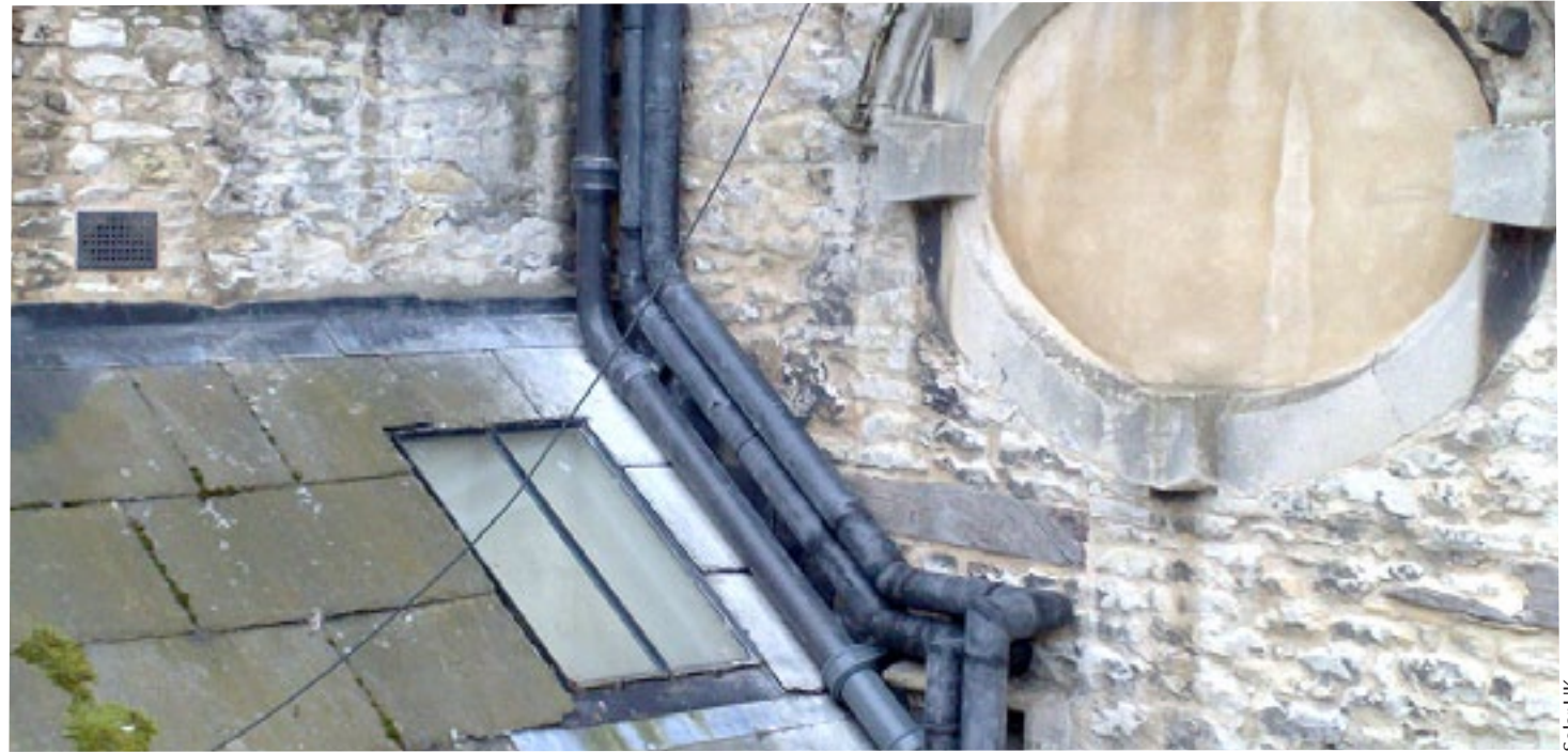
Above Distribution pipework from roof collectors to hot water cylinder
